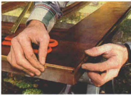
Head strip gets notched. A small notch is cut out of the door's head strip to mate with the jamb strip on the hinge side.
